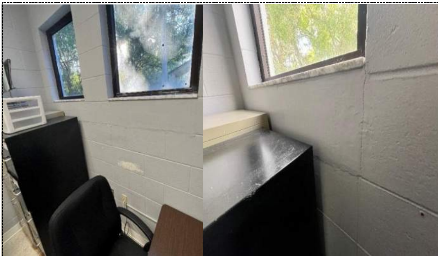
Photo 80 - Evidence of repairs/infills in kitchen managers office-building 3.
