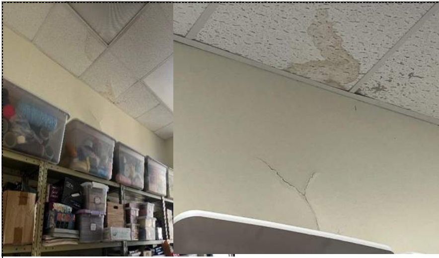
Photo 52 - Water stained ceiling tiles and wall damage in Art room closet-building 1.
