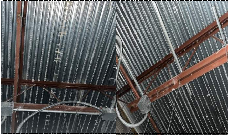
Photo 102 - Evidence of roof leaks above ceilings in classrooms-building 2.
