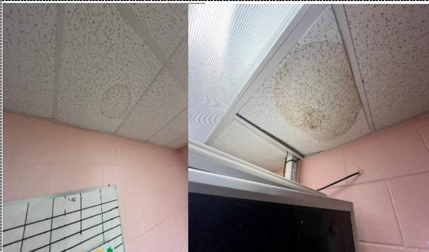
Photo 74 - Water staining on ceiling tiles in PE office-building 3.
