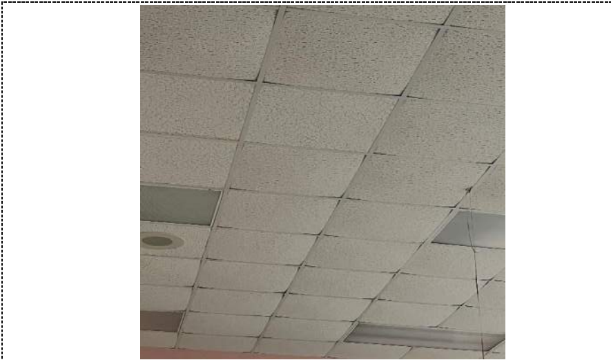
Photo 64 - Ceiling tiles bowed throughout Cafeteria-building 3.
