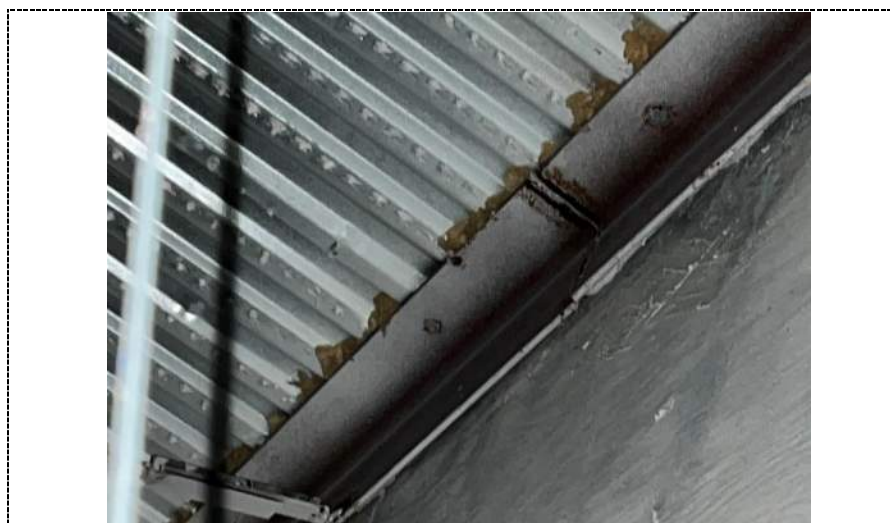
Photo 104 - Evidence of above ceiling roof leaks along parapet wall in Northwest classroom in North pod (stained ceiling tile below)- building 2.
