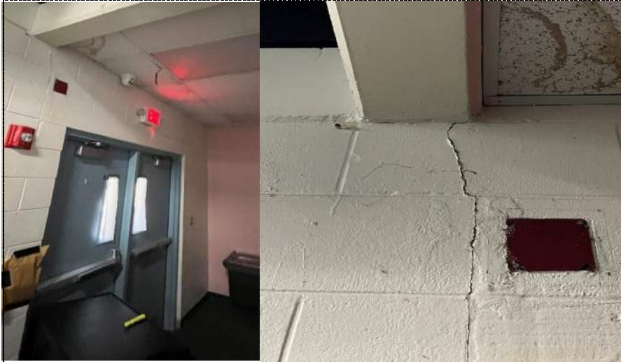
Photo 66 - Water staining ceiling tiles and cross block cracking at end of hallway along Northeast side of Cafeteria-building 3.
