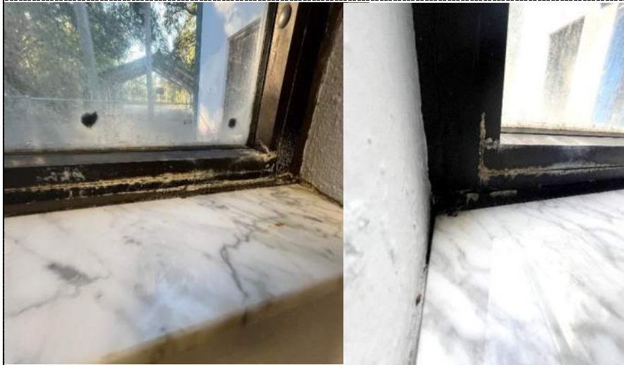
Photo 81 - Evidence of window leaks in kitchen managers office-building 3.
