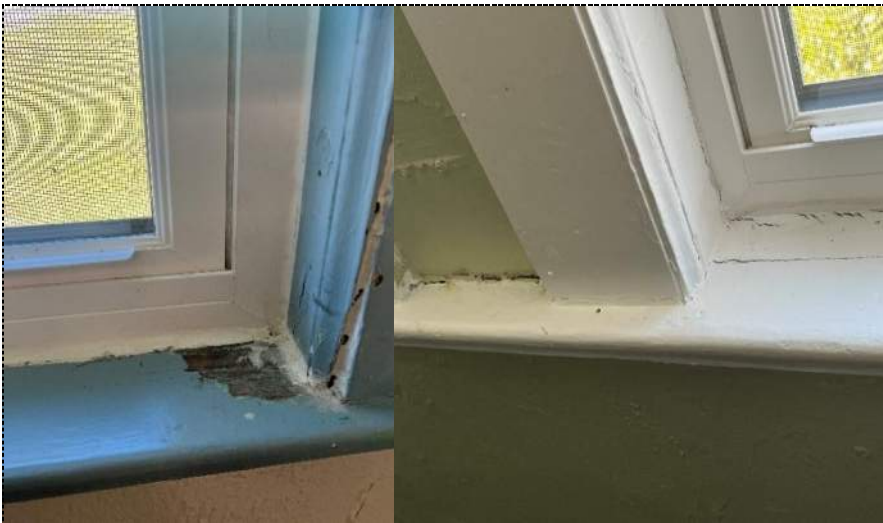
Photo 22 - Evidence of water intrusion and wall damage along exterior wall on admin side of building 1.
