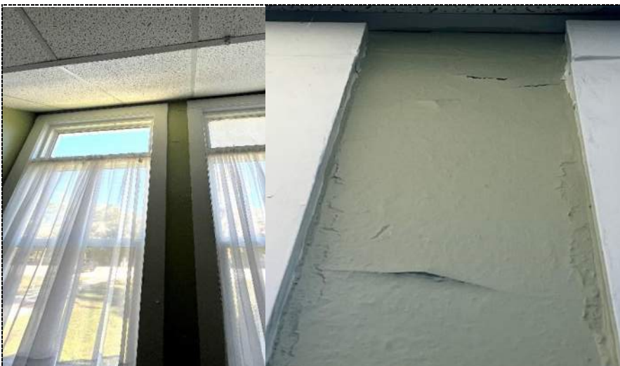
Photo 23 - Evidence of water intrusion and wall damage along exterior wall on admin side of building 1.
