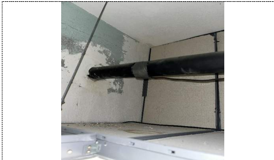
Photo 16 - Source of above ceiling leak in center office in hallway leading to break room in building 1..
