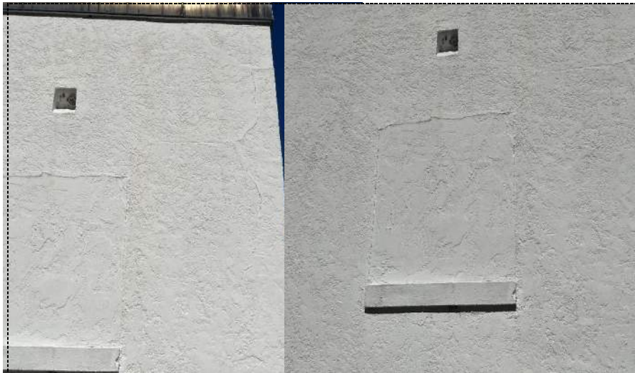
Photo 4 - Infill and exterior cracking at Southeast corner of building 1 break room (interior damage).
