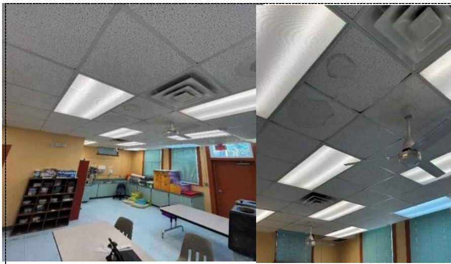
Photo 26 - Water stained ceiling tiles in the conference room-building 1.
