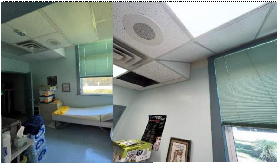
Photo 13 - Evidence of roof leaks, wall damage and possible microbial amplification above ceiling in first office on South side of building 1.
