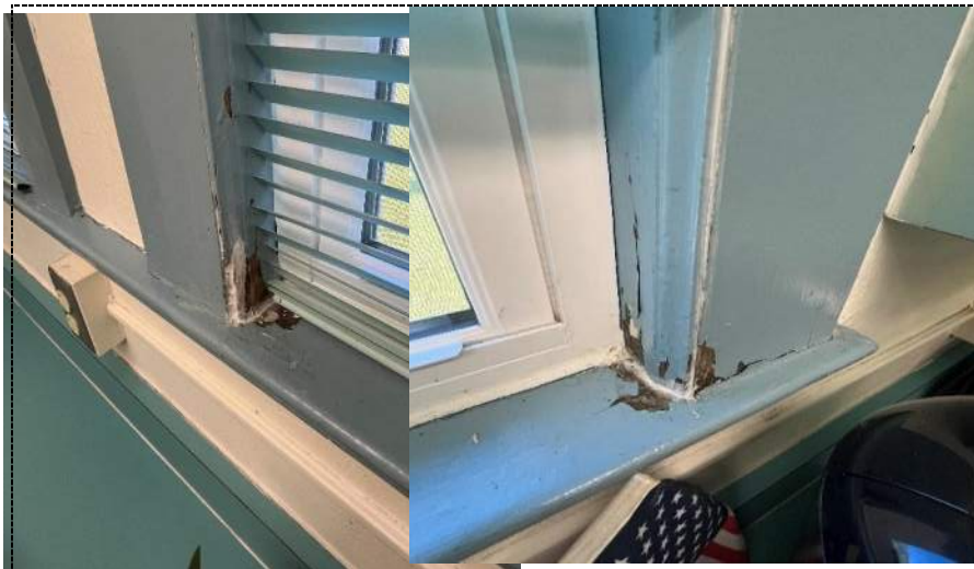
Photo 20 - Evidence of water intrusion and wall damage along exterior wall on admin side of building 1.
