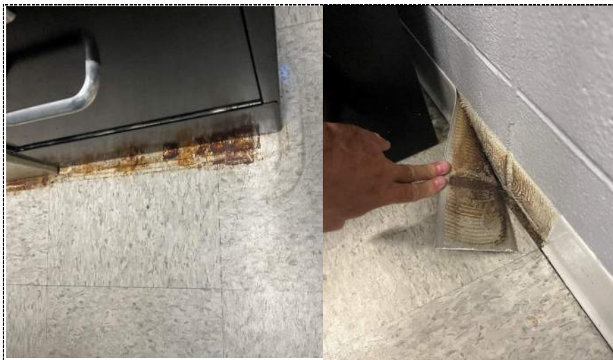
Photo 83 - cabinets and peeling cove base in the kitchen managers office-building 3.
