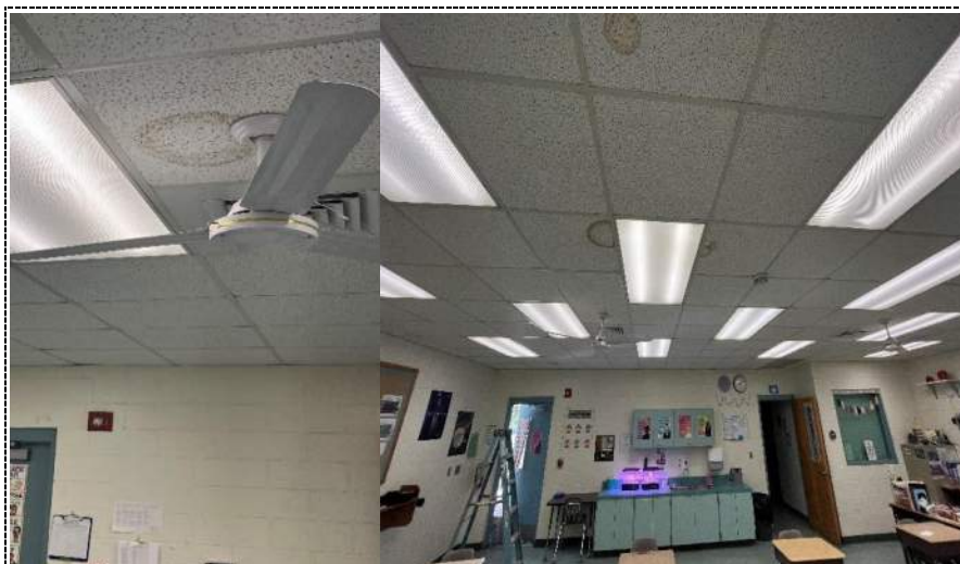
Photo 95 - Water stained ceiling tiles throughout North and South classrooms- building 2.
