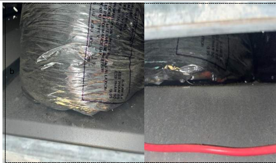
Photo 30 - Poorly sealed diffusers in conference room - building 1.
