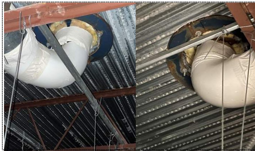
Photo 101 - Evidence of above ceiling leaking rain leaders in classrooms-building 2.
