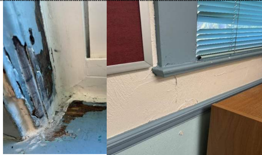
Photo 21 - Evidence of water intrusion and wall damage along exterior wall on admin side of building 1.
