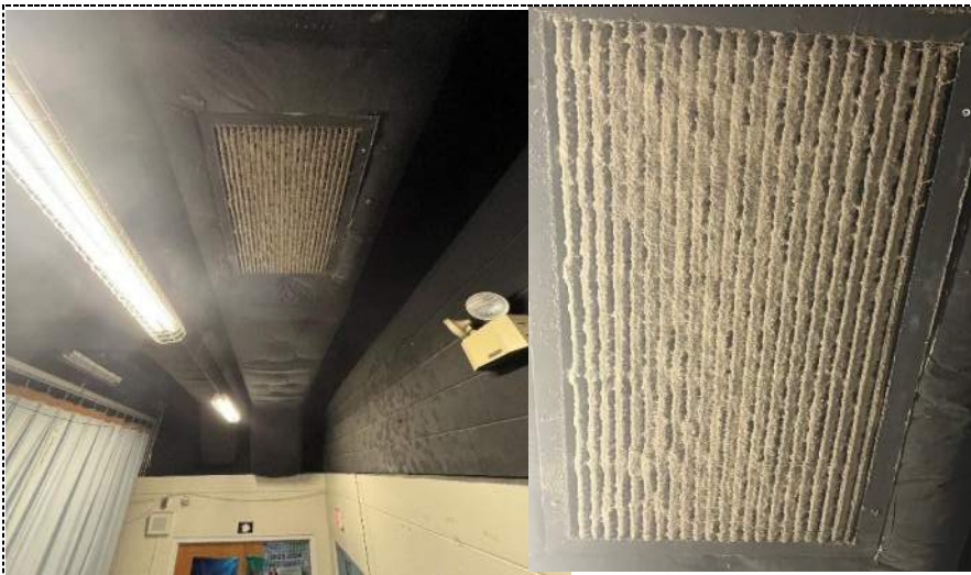
Photo 70 - Very dirty HVAC grate and possible microbial amplification on North wall behind stage outside of PE office-building 3.
