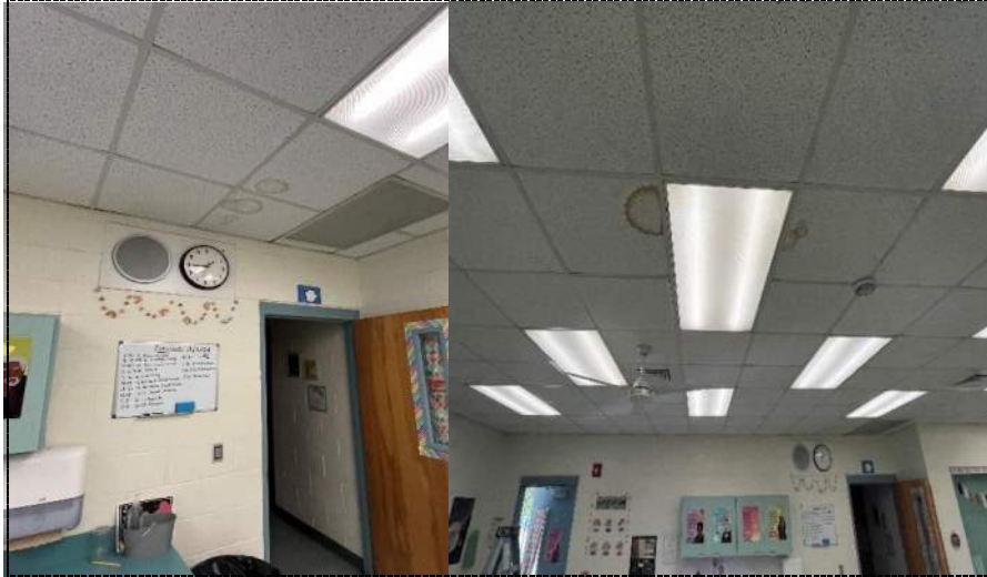
Photo 96 - Water stained ceiling tiles throughout North and South classrooms-building 2.
