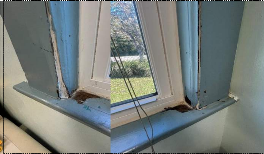
Photo 24 - Evidence of water intrusion and wall damage along exterior wall on admin side of building 1.
