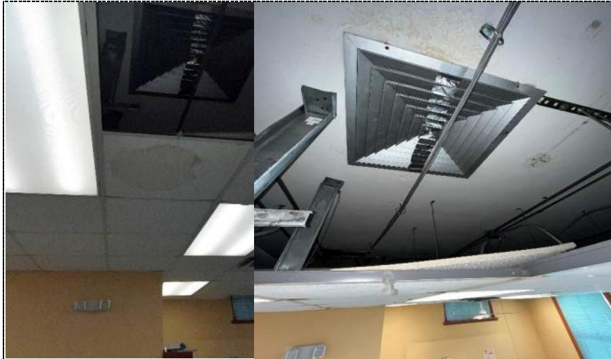
Photo 27 - Possible active and sweating diffuser above the drop ceiling in conference room-building 1.
