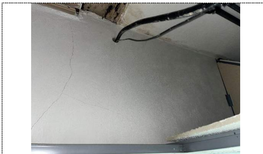
Photo 14 - Wall damage and possible microbial amplification above ceiling in first office on South side of building 1.
