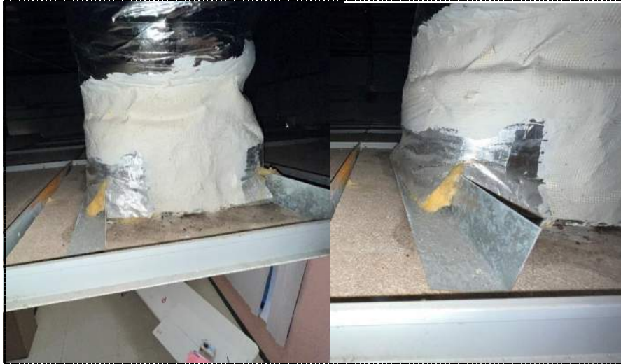
Photo 90 - Poorly sealed diffuser with evidence of moisture impact on the back of surrounding ceiling tiles in room to the Southwest corner of Cafeteria-building 3.
