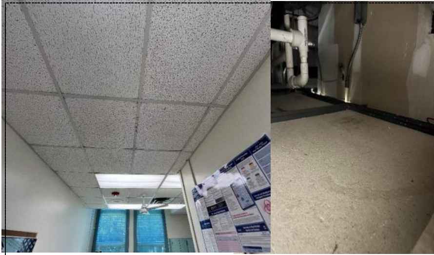
Photo 18 - Slight water staining on ceiling tile below air handler in break room -building 1.
