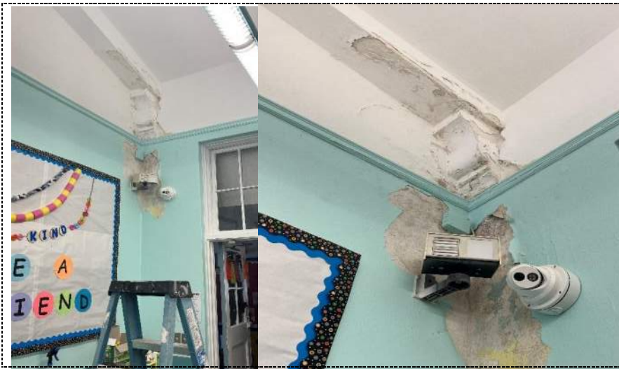
Photo 37 - Water damaged walls with microbial amplification in Media room- building 1.
