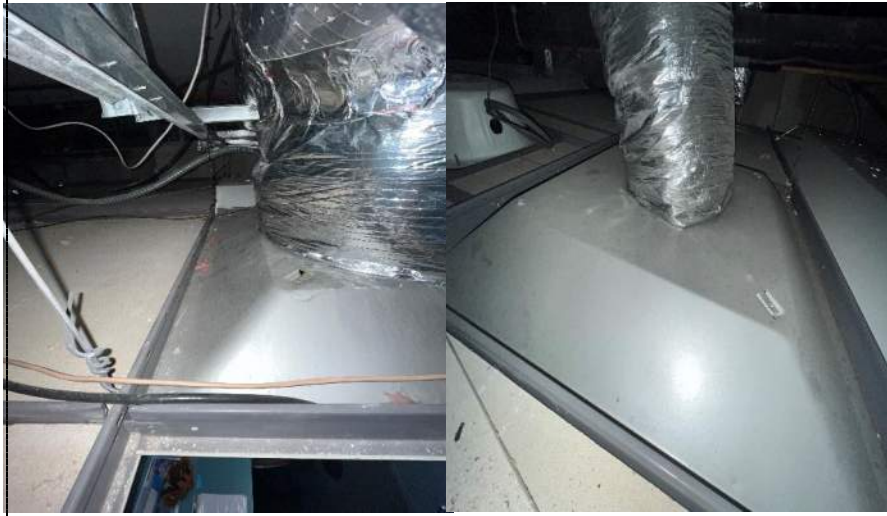
Photo 12 - Poorly sealed duct to diffusers connection- building1.
