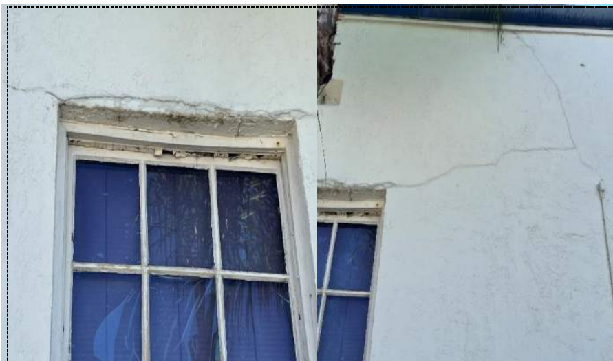
Photo 5 - Exterior wall cracking and window seal deficiencies- building 1.
