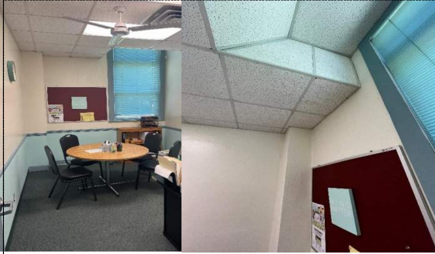
Photo 15 - Evidence of above ceiling leak in center office in hallway leading to break room in building 1.
