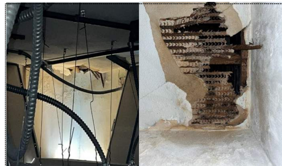
Photo 32 - Collapsed ceiling above drop ceiling with evidence of roof leak in conference room - building 1.
