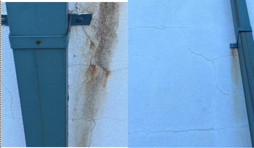
Photo 58 - Wall damage next to downspouts-building 3.
