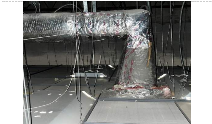
Photo 100 - Poorly sealed diffusers in classrooms-building 2.
