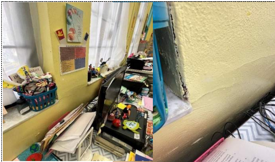
Photo 49 - Evidence of wall damage of Art room-building 1.
