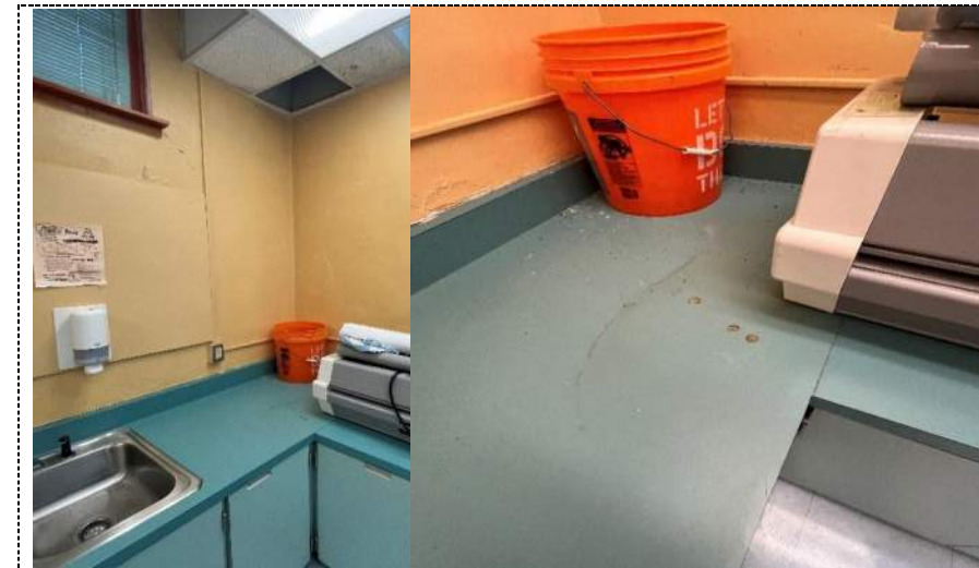
Photo 31 - Collapsed ceiling tile with catch bucket and water staining on countertop in conference room - building 1.
