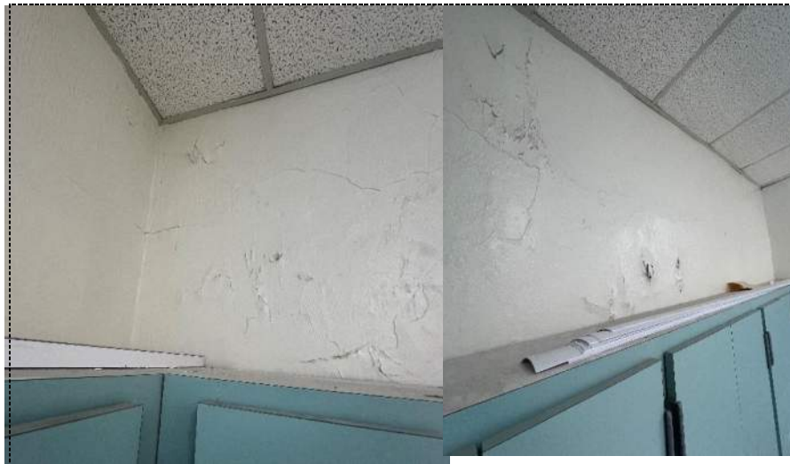
Photo 19 - Wall damage in Southeast corner of break room corresponding to Southeast exterior infill-building 1.
