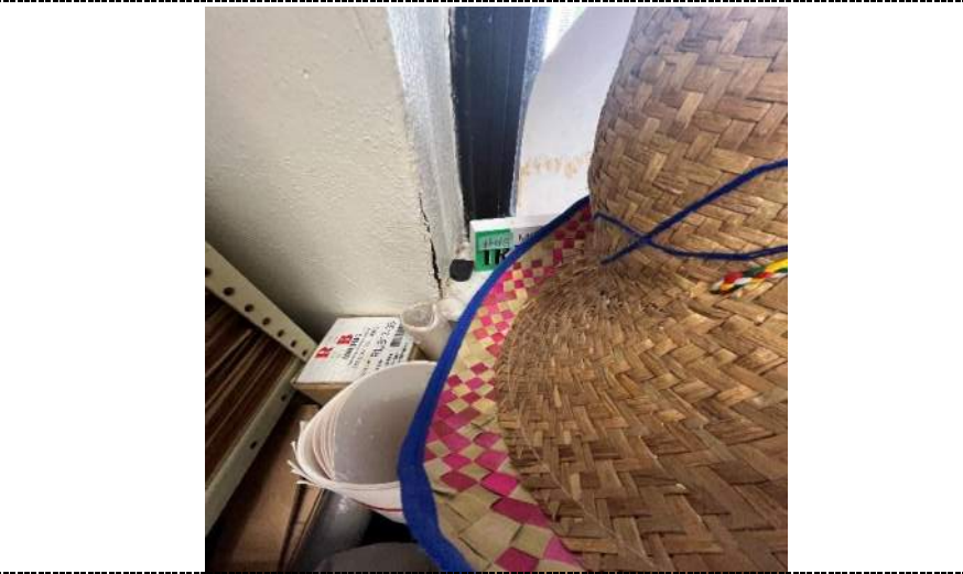
Photo 55 - Evidence of damage around window in Art room closet-building 1.
