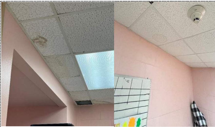
Photo 85 - Water stained ceiling tiles in room to the Southwest corner of Cafeteria-building 3.
