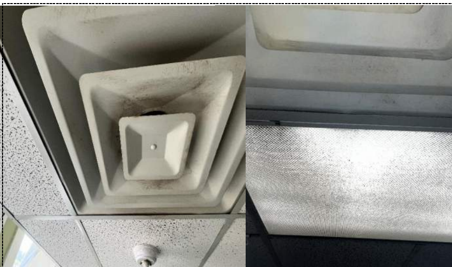
Photo 11 - Casting and possible microbial amplification on diffusers throughout admin area-building 1
