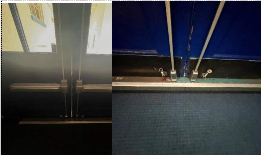
Photo 43 - Poorly sealed exterior doors- building 1.
