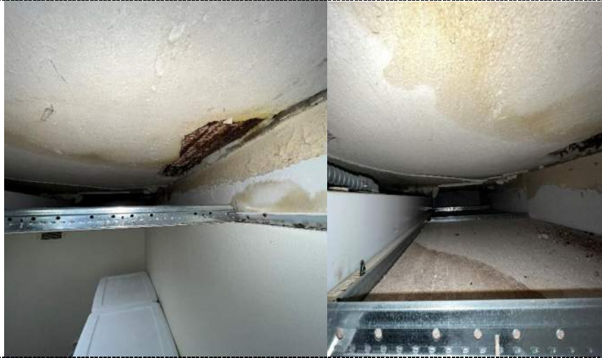
Photo 54 - Evidence of roof leak above ceiling in Art room closet- building 1.
