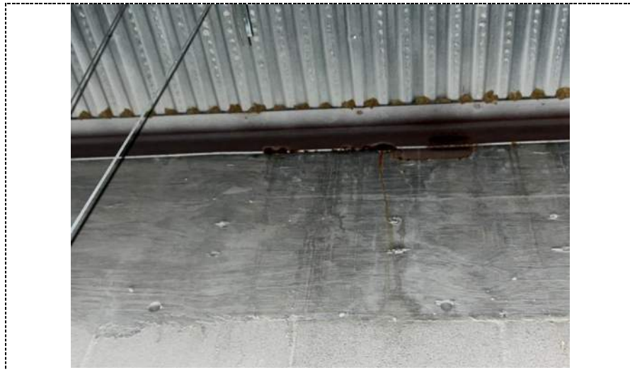
Photo 103 - Evidence of above ceiling roof leaks along parapet wall in Northwest classroom in North pod (stained ceiling tile below)- building 2.
