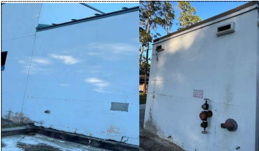
Photo 59 - Exterior cracking and areas of failing weatherproofing around building-building 3.
