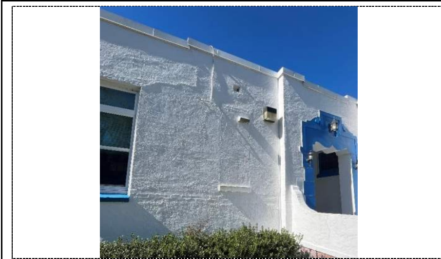
Photo 3 - Infill and exterior cracking on front elevation-building 1.
