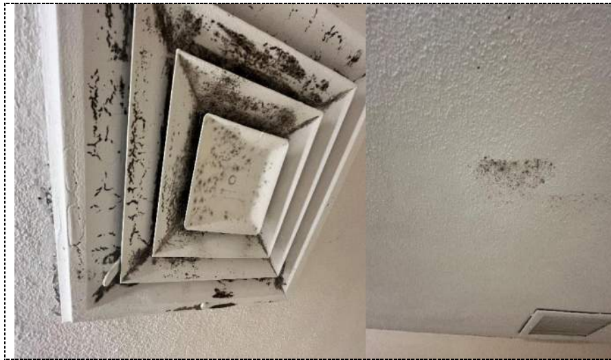
Photo 40 - Casting and microbial amplification on diffuser and ceiling in office behind Media room-building 1
