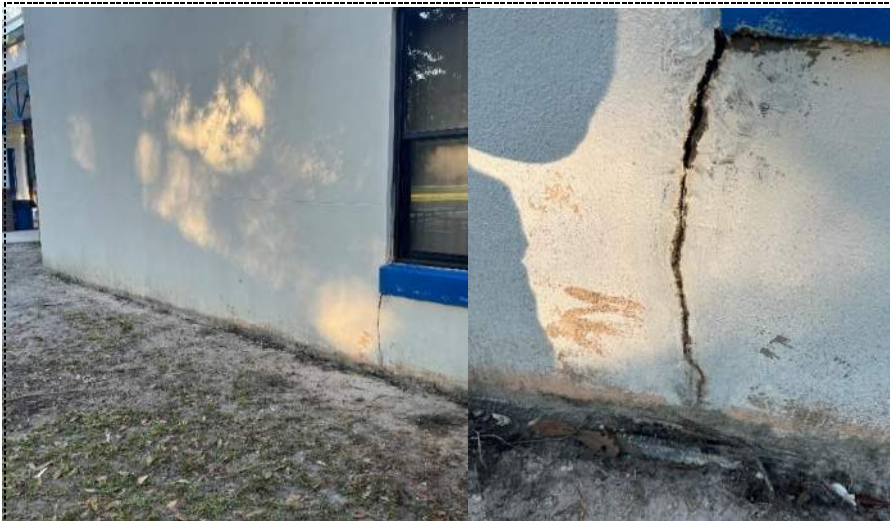
Photo 61 - Exterior structural crack with interior damage in Southwest corner of Cafeteria-building 3.
