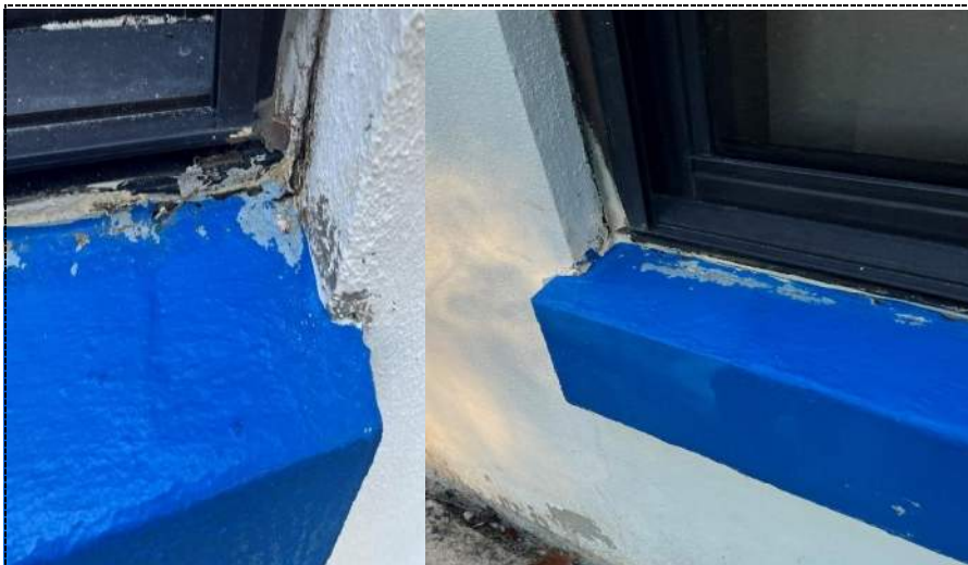
Photo 62 - Evidence of window seal deficiencies-building 3.
