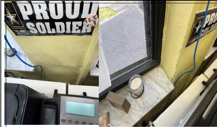
Photo 48 - Evidence of wall damage of Art room-building 1.
