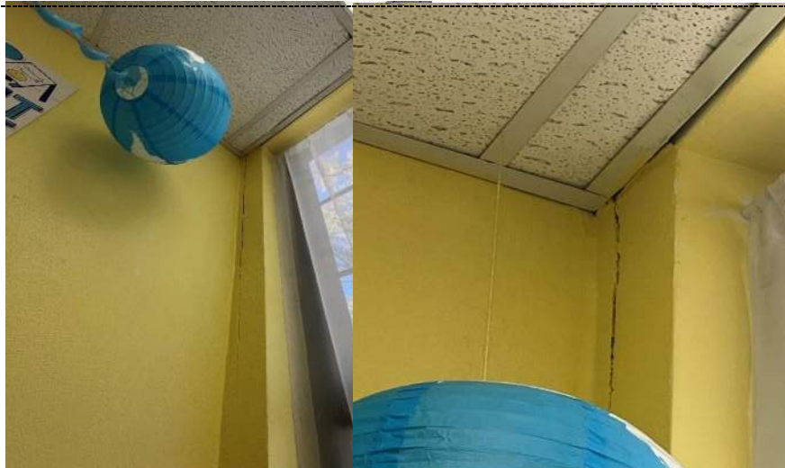
Photo 50 - Structural crack in Northwest corner of Art room- building 1.
