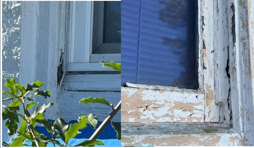
Photo 6 - Window seal deficiencies and wood rot- building 1.
