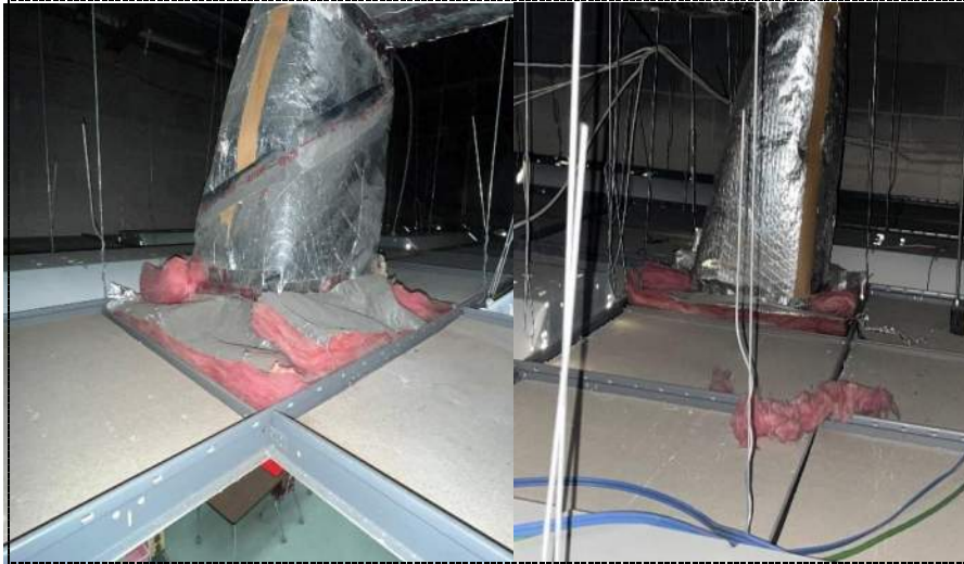
Photo 99 - Poorly sealed diffusers in classrooms-building 2.
